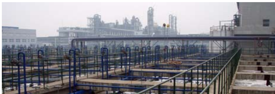
Waste-water treatment at a Chinese supplier.
