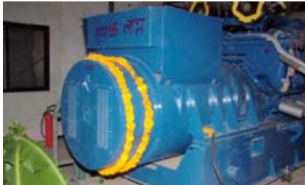
Gas engine, Cheminova India.
