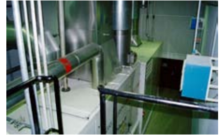
Gas turbine, Cheminova DK.
